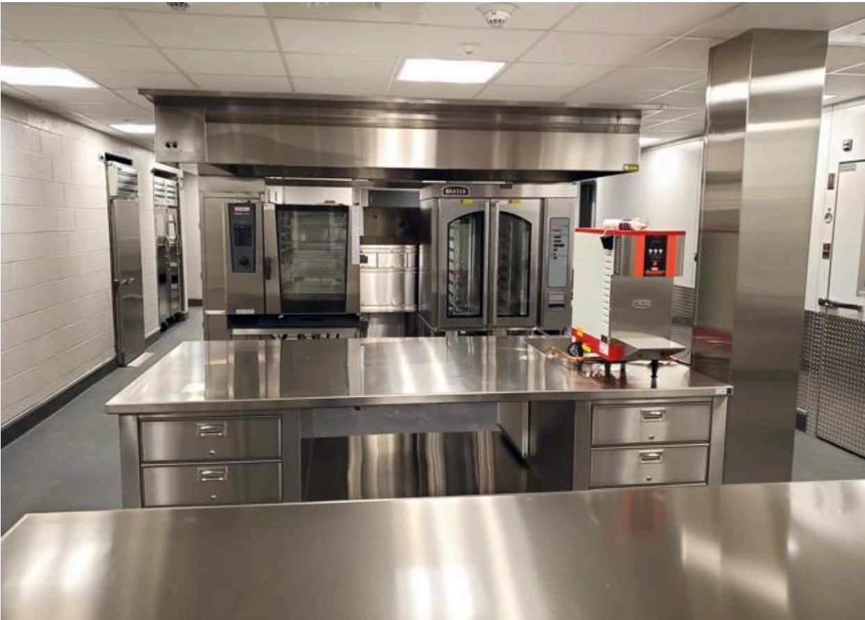
Double-wide stainless-steel tables contain no overshelves. Below, storage on undershelves and tiered drawer systems maximize sightlines through the kitchen.
